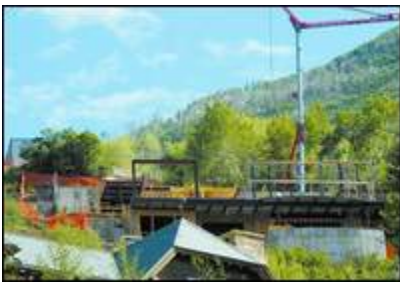
Pitkin County's public works director plans to ask the county commissioners to hold off on a $2 million road project on Red Mountain until the construction is complete. (Mark Fox/The Aspen Times) Click to Enlarge
